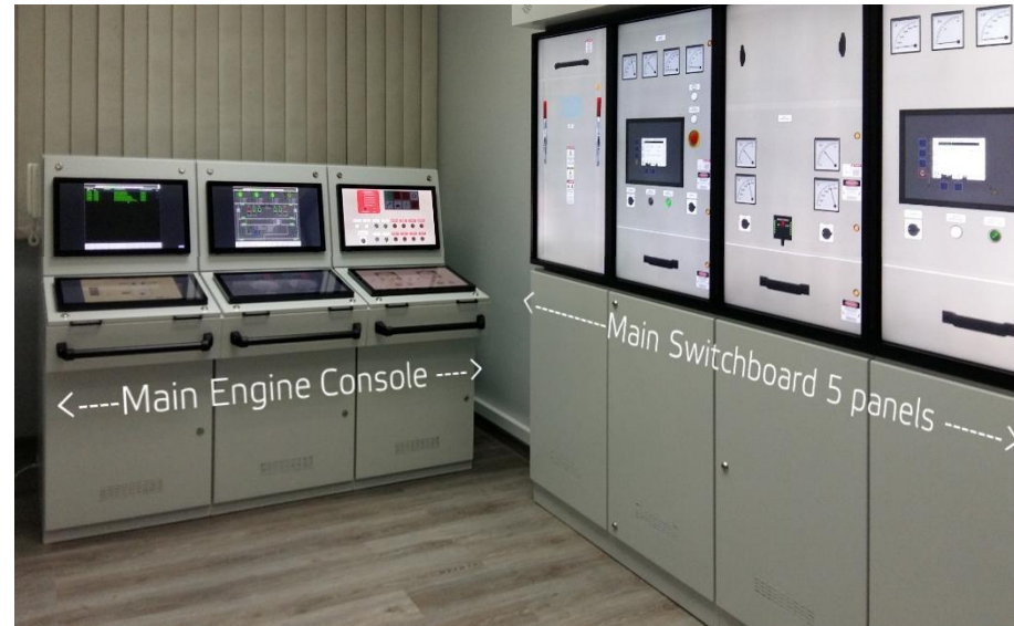
Full Mission Simulator – example of arrangement of the main Engine Console and the Main Switchboard in the Engine Control Room
